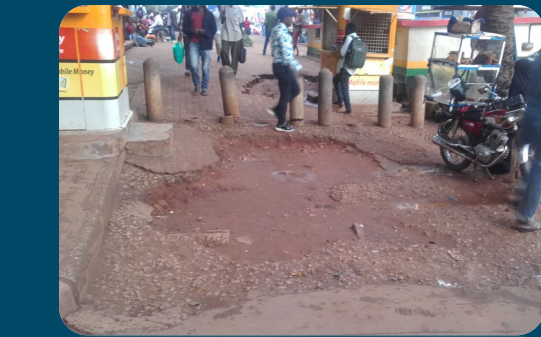
A blocked walkway in Kampala. Photo credit: CEBHA
